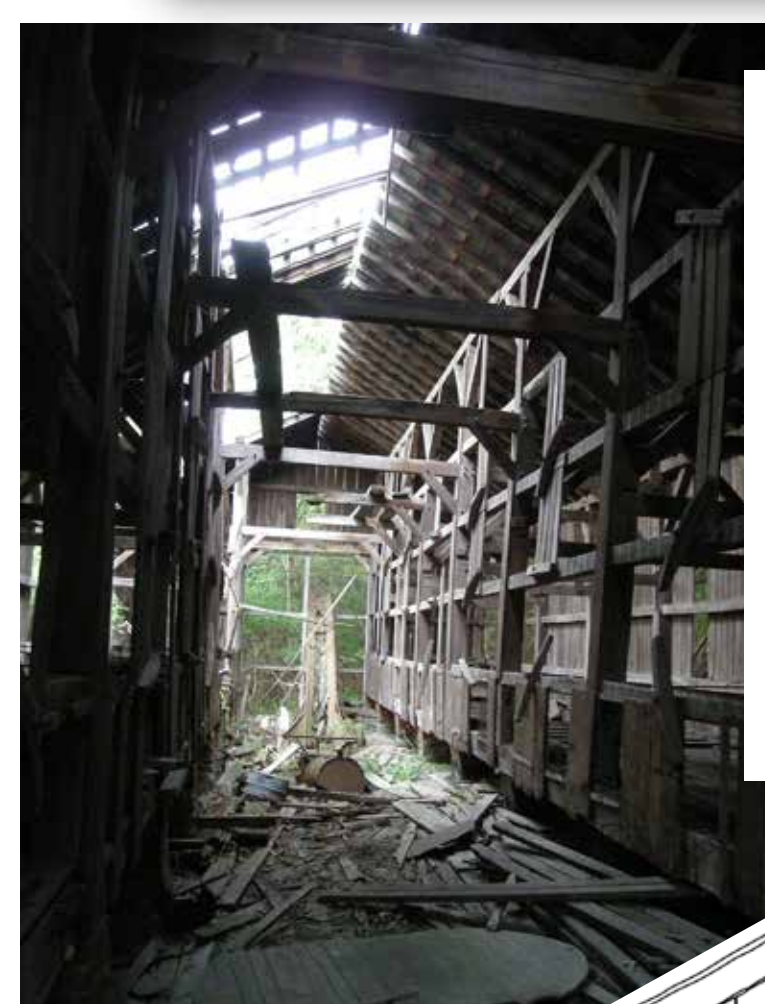
Interior of corn crib showing damage.
